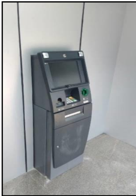
Picture 2 ATM in False wall
