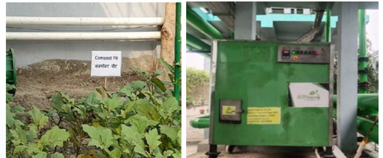
Compost pit and machine installed for the recycling of waste at SBIL, Kolkata
