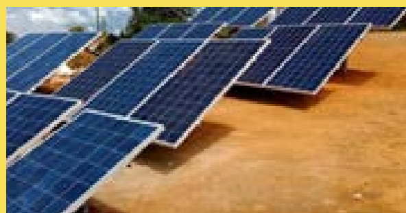
Solar installation under the initiative at Pungro Branch in the Bank's North East Circle
